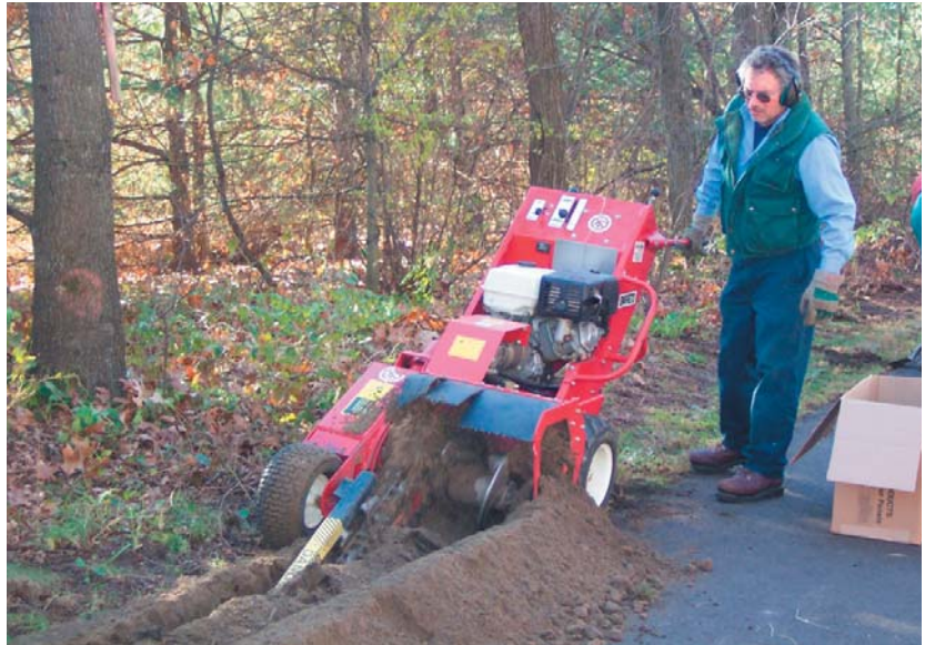
Volunteer Peter Brooks guides the "Ditch Witch" alongside the Manhan Rail Trail during a recent work party. The machine cut a deep narrow ditch so that a thick vinyl root barrier could be installed.
